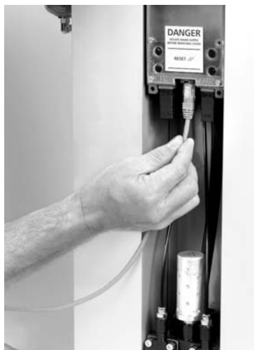
Connecting the PC to the controller
